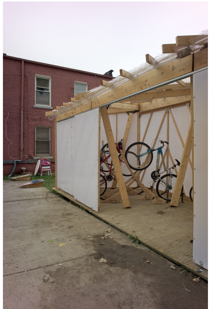
Figure 1. Project installed at Hostel Detroit
